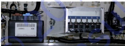
Fault Box and BCM installed on rear of CL-1918-02B
