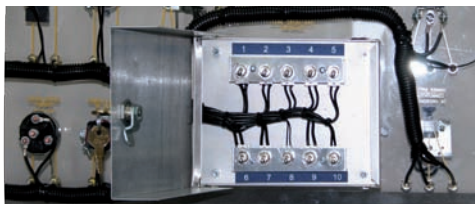
CL-1918-02 (rear view with fault box opened)
